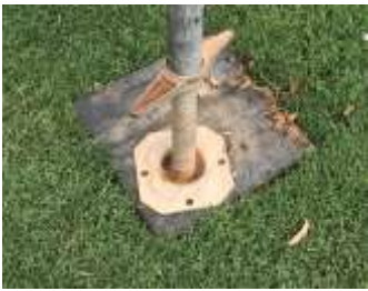
Sole plate in unacceptable condition 1
